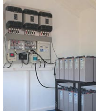
meeco sun2com installation -Battery & inverter room
