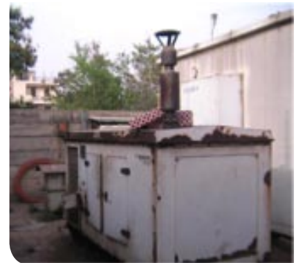
Diesel Generator example, India
